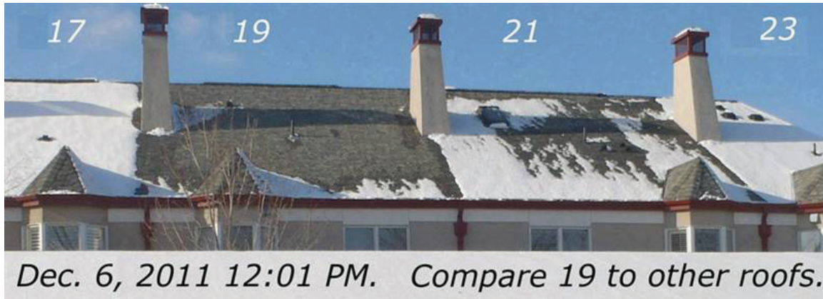
FIGURE 7: Townhouse roof snow melt patterns reveal heat loss. Reprinted from (C) HankeyandBrown.com.
