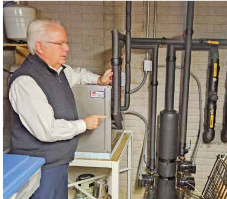
John Forbes had a geothermal heat pump installed.
