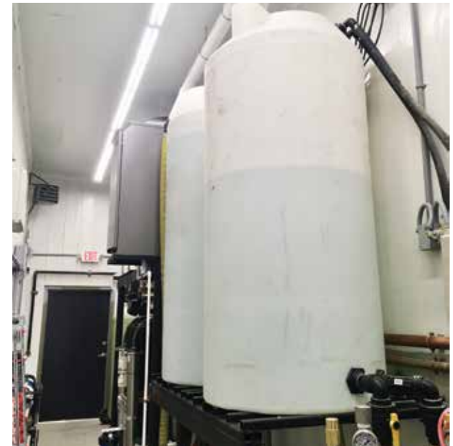
Two large water tanks are included in the utility room between the two bays. One holds water directly from the Panora water system. The other holds water that has been channeled through both water softener and reverse osmosis equipment to produce "spot free"
