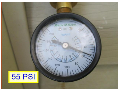
E. Item 1(Picture) water pressure info
