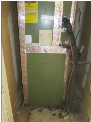
A. Item 1(Picture) FAU closet garage
