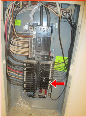
B. Item 1(Picture) sub panel master bedroom closet
