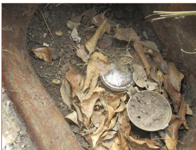
E. Item 2(Picture) water meter
