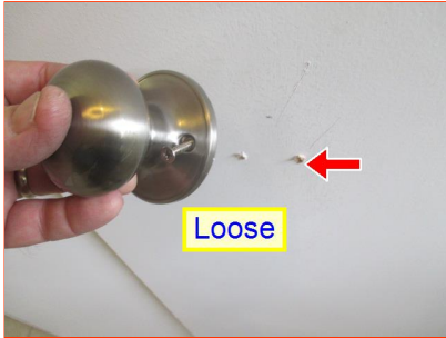
G. Item 1(Picture) laundry room handles
